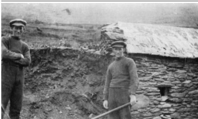
Paddy and Maurice Keane demolishing their old house. This was the house of their maternal great grandfather, the poet Seán Ó Duinnshléibhe
